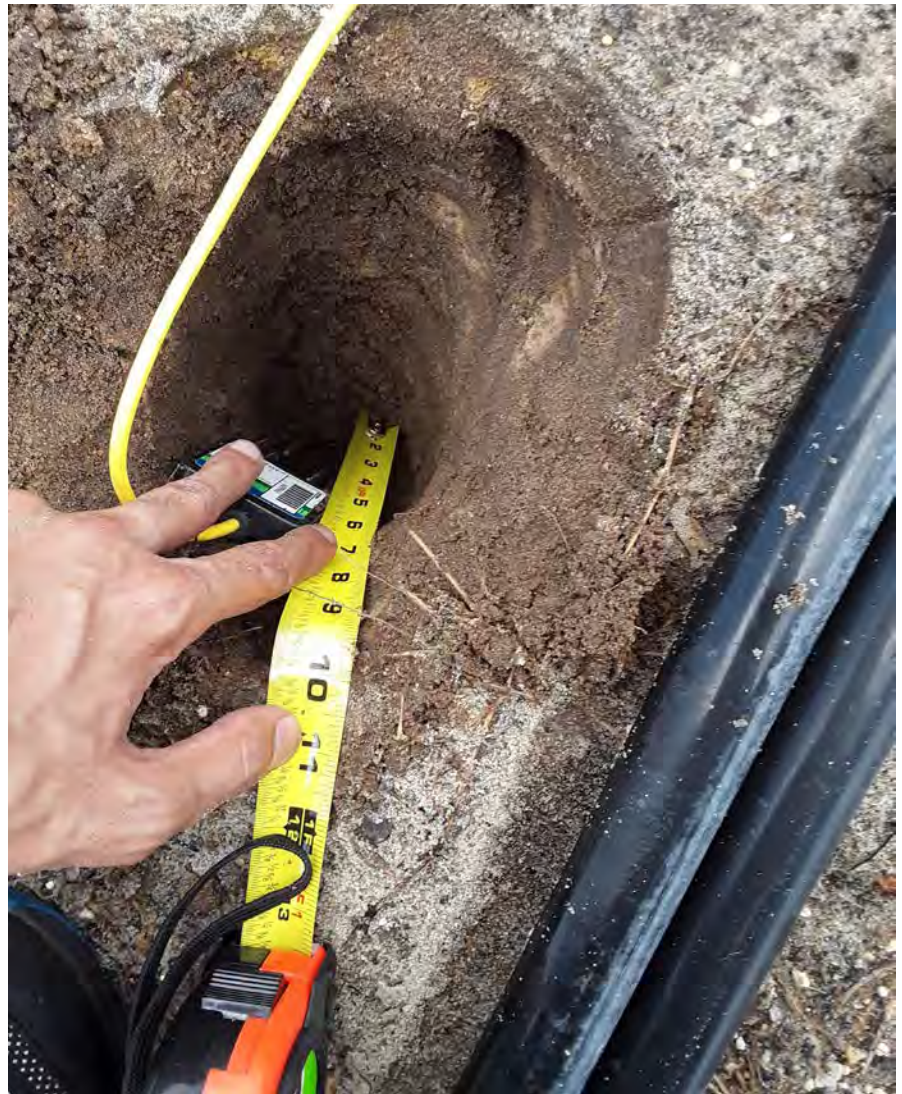
A soil moisture sensor is installed vertically.
