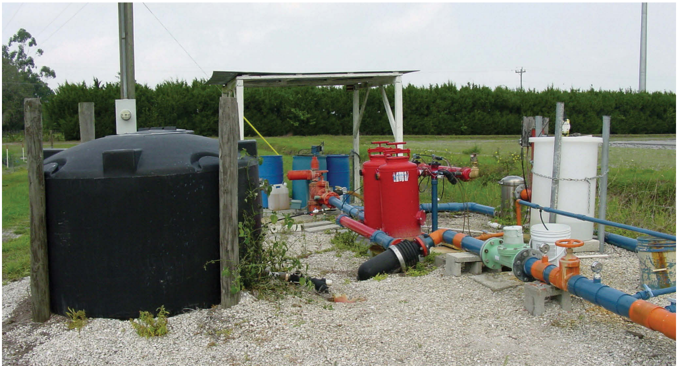
Figure 1. Fertigation system including backflow prevention devices
